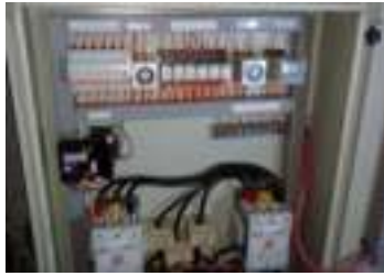
Gambar 5. 65 Generator set (auto switch system)
