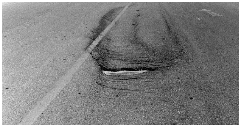
Gambar 2.6. Retak slip ( slippage cracks )
