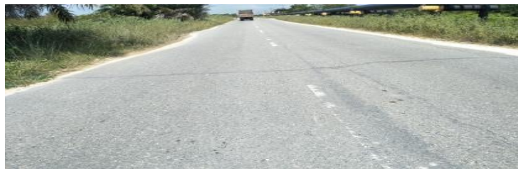
Gambar 2.8 Retak Melintang ( Transversal Cracks )
