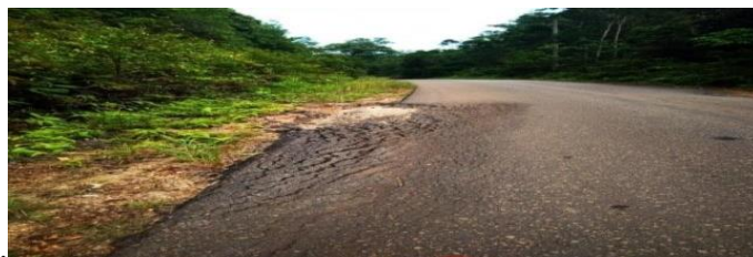
Gambar 2.6 Cacat Tepi Perkerasan ( Edge Cracking )
