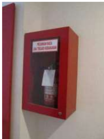
Gambar: fire extinguisher
